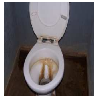
Stained plumbing fixture by groundwater.
